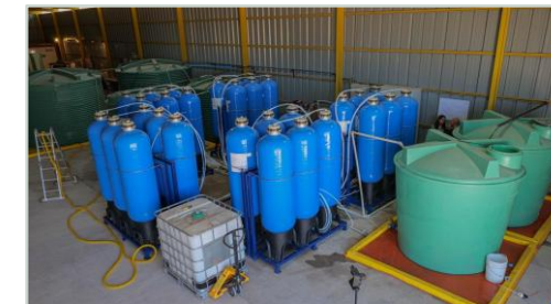
the 1 t/month pilot plant, Copiapó
