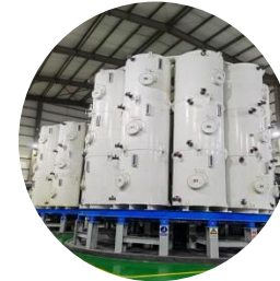
Existing DLE plant, Xi'an, China
